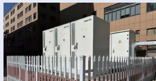
金盛服饰1.075MWh-工商业储能
